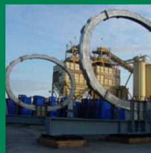
O-shaped rings form a base for the pipe truss system and plates erected by MTH.
