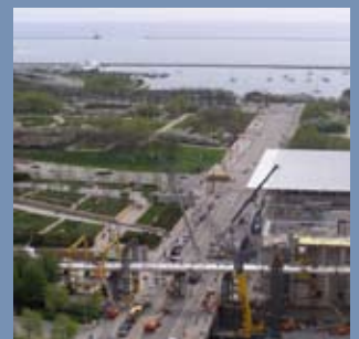
Danny's Construction crane operated from a busway below Monroe St. and lifted the 110,000-lb section to cross it.
