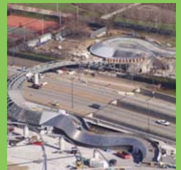
Imperial Construction Associates erected the sections over Columbus Drive in one weekend. Cladding was done by Permasteelisa and Radius Track.
