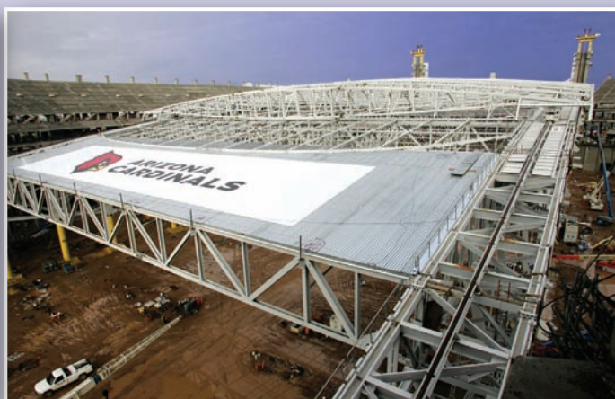
2007 IDEAS 2 National Winner – 400 tons of 12 inch square tubing curved for the retractable, lenticular roof trusses. The University of Phoenix Stadium. Phoenix, AZ.
